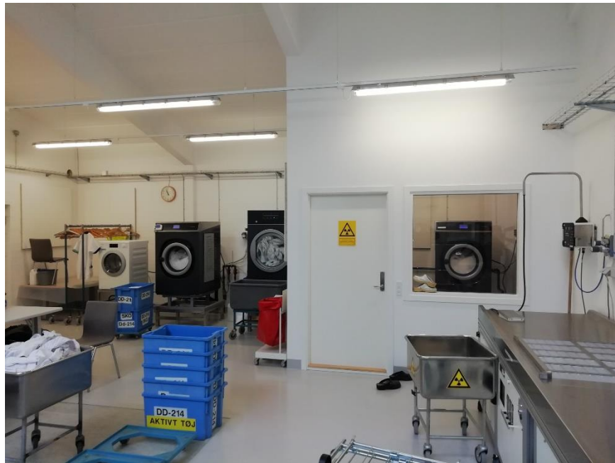
Figure 36: The laundry facilities, including the active laundry in its new location in Building No. 217.
