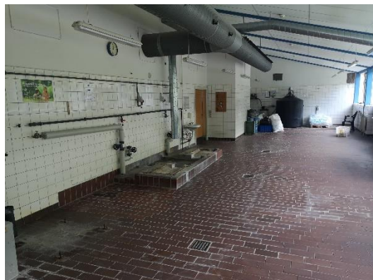
Figure 35: The laundry, including the active laundry area to be prepared for contamination survey
