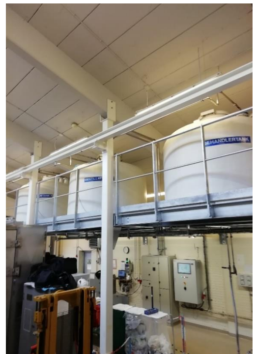
Figure 38: New steel deck above the distillation unit for the associated tank in Building 217.
