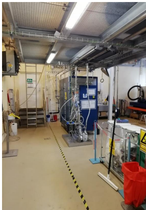
Figure 37: New location of the distillation unit in Building No. 217 with the associated tanks placed above on an inserted steel deck.
