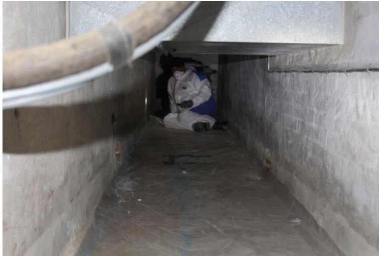
Figure 31: Crawlspace with uranium contamination in the floor
